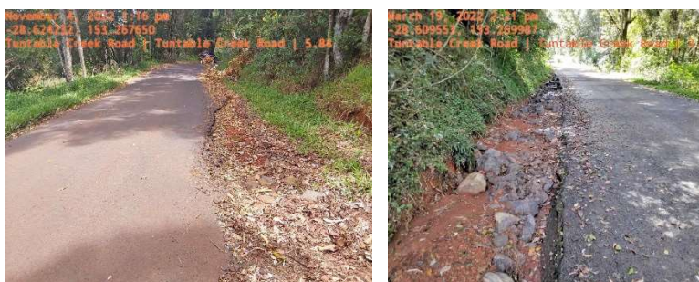
Tuntable Creek Road – Damage after Natural Disaster
