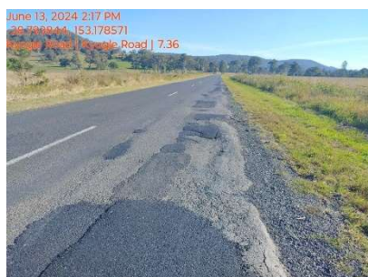
Damage after Natural Disaster
