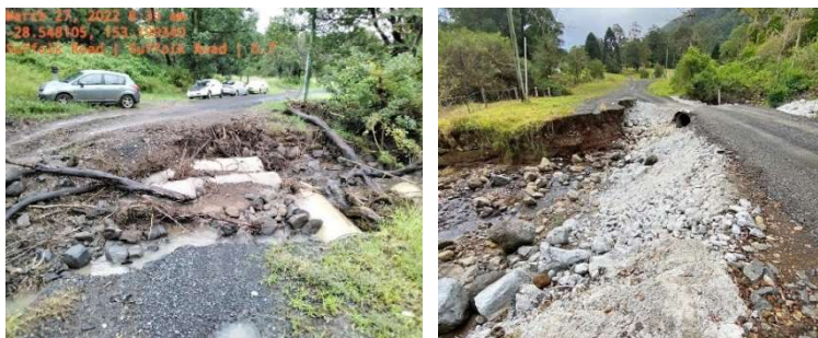
Suffolk Road – Damage after Natural Disaster
