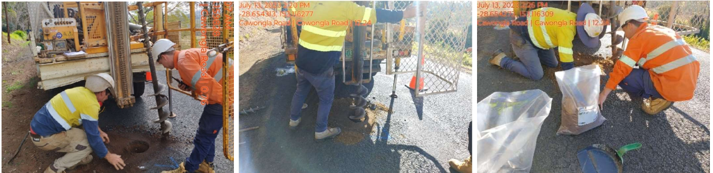
Pavement Investigations on Cawongla Road
