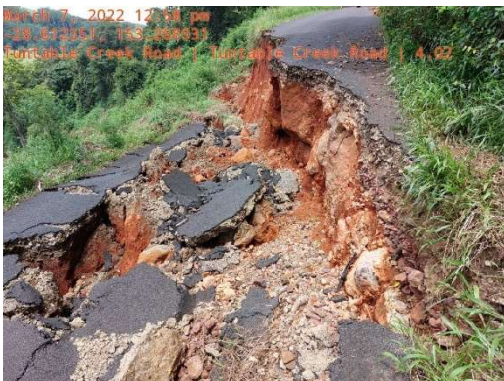
Image: Image of embankment failure before restoration works
