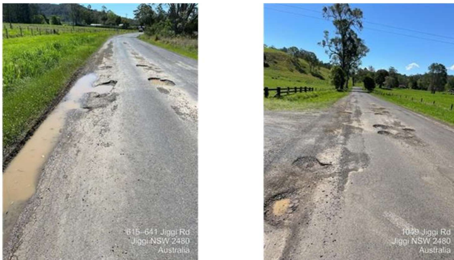
Image: Jiggi Road flood damage
