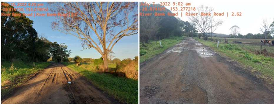
Image: Riverbank Road flood damage
